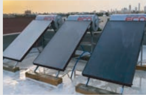
Solar Water Heater
